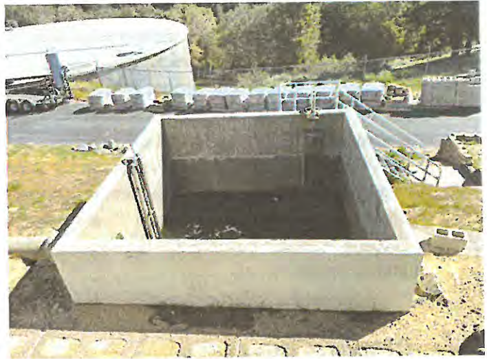
Figure 5. Existing Diversion Box to Emergency Storage Reservoir
